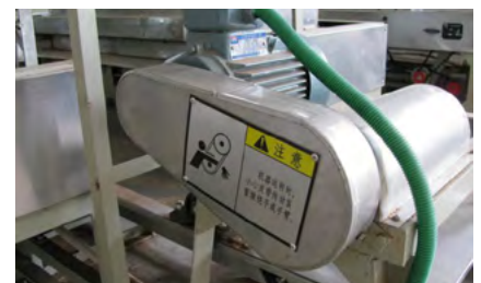
Machinery with safety guard & clear hazard sign
