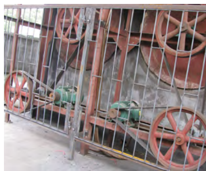
Guarded machine: good practice demonstrated in the toolkit
